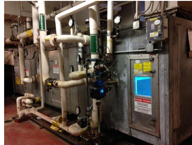
Existing HVAC AHU-2 in West Mechanical Room
