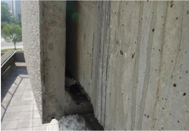
View of Exterior Panel and Cavity without a Vapor Barrier and Insulation
