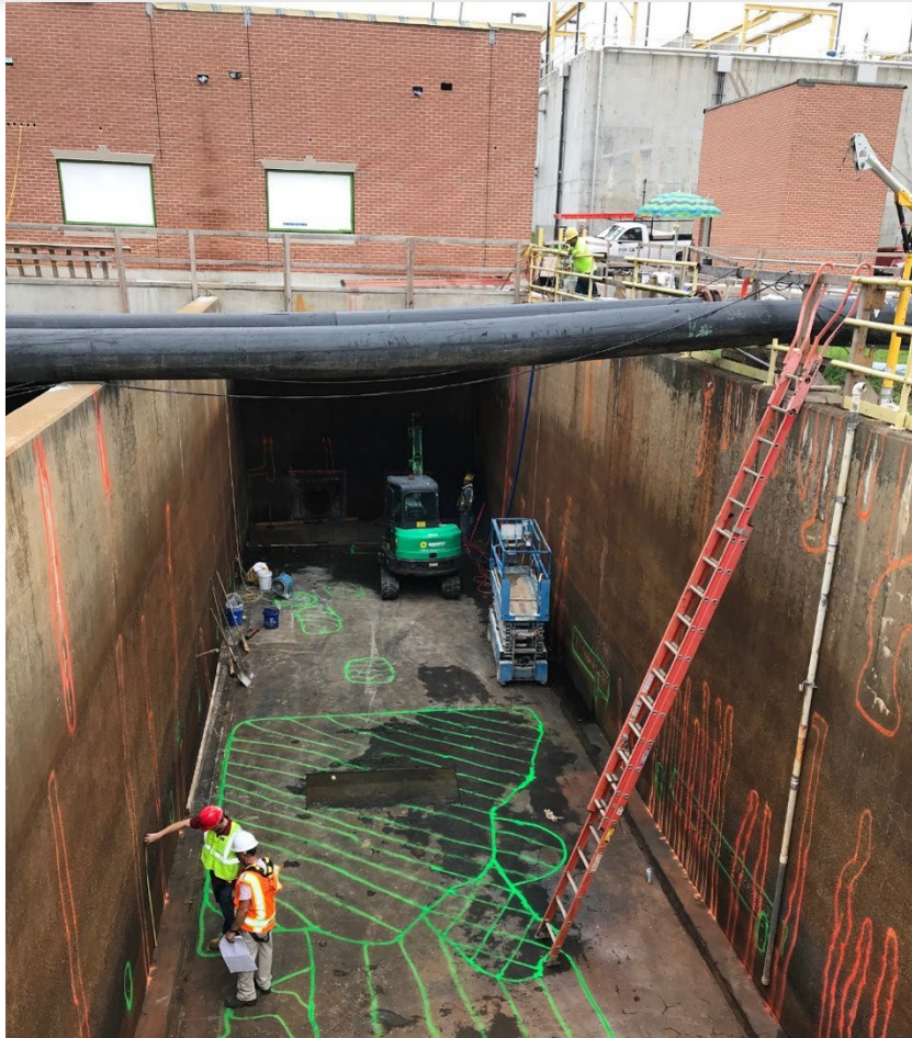
Noman M. Cole Jr. Pollution Control Plant Tertiary Filters
