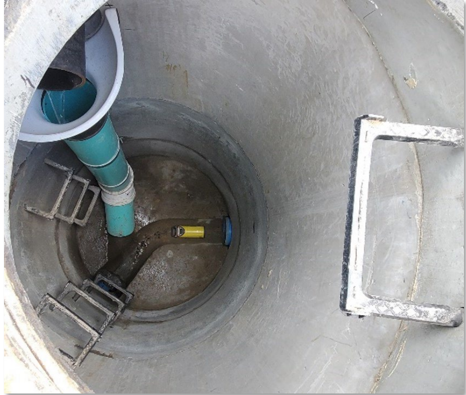
Fort Hunt Gravity Sewer
