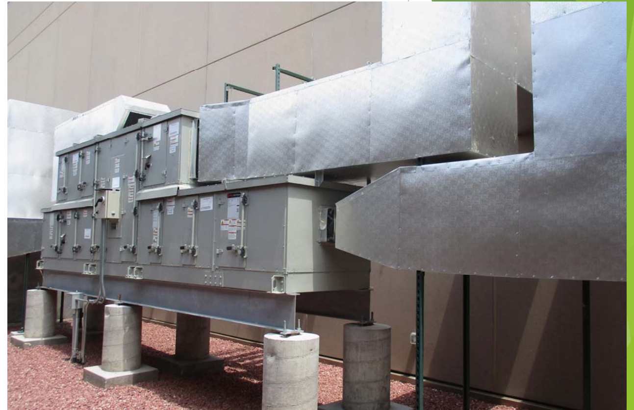
Exterior mechanical yard with air handling unit, placement provides excellent clearance for maintenance
