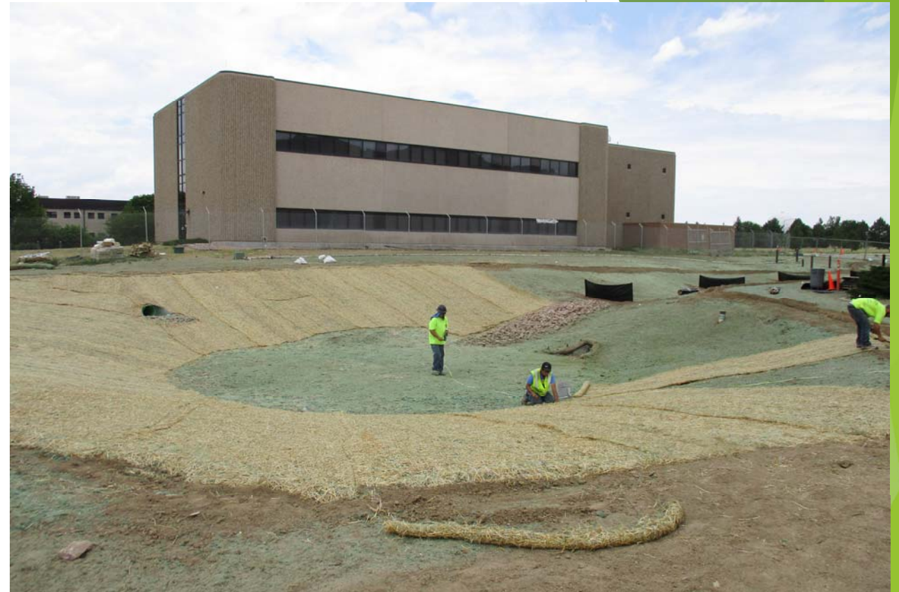
Sand Filter Extended Detention Basin Retained the entire volume of the 1-year and 2-year post-development runoff, reducing the peak runoff from those events to zero.
