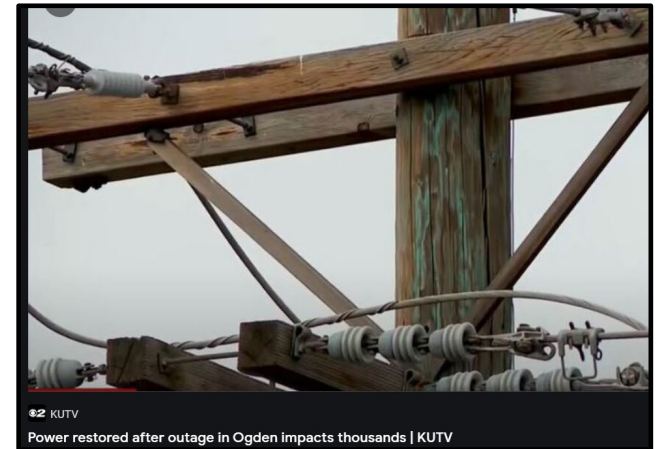
Weather and infrastructure increase risk of commercial power outages
