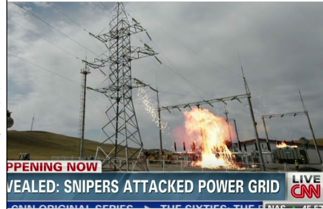
Large transformers damaged by unknown attackers in CA Source: CNN
