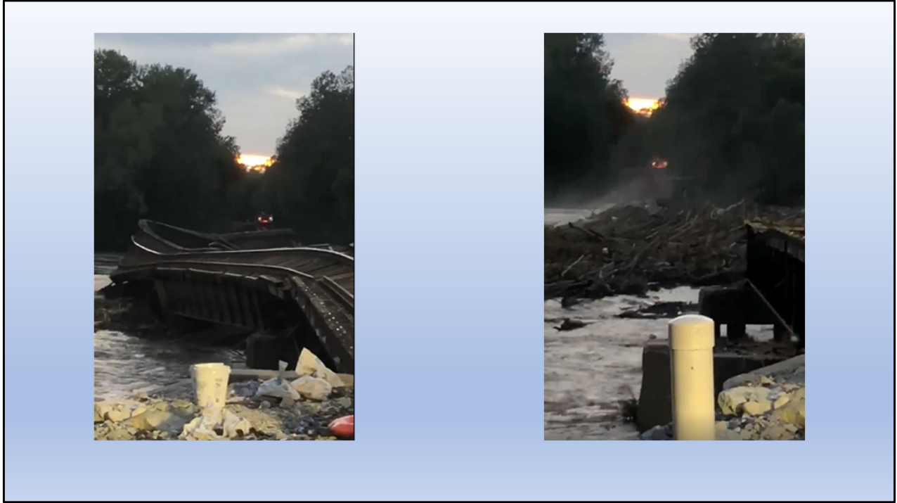
Image clips from the video as the bridge fails and the log jam rushing through the opening
