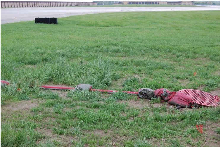
Exposed Airfield Wiring
