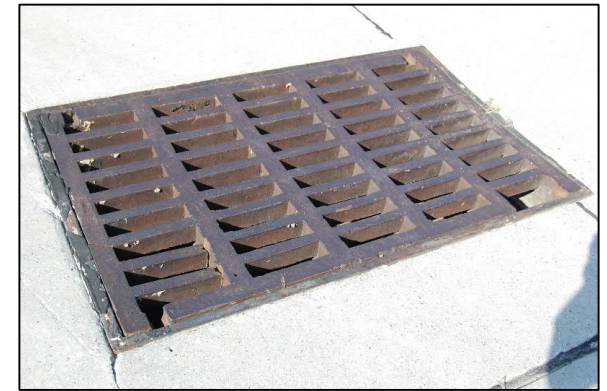
Broken Drainage Infrastructure
