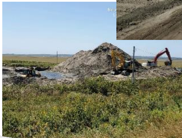
Above and to Right: Progress of levee work and proximity of alternate sand borrow source at Fox Lake. Dredging of sand at Fox Lake is shown above with placement of sand seepage berm at the right.
