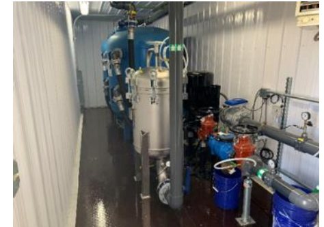
Inside Mobile (Conex) IX Treatment System
