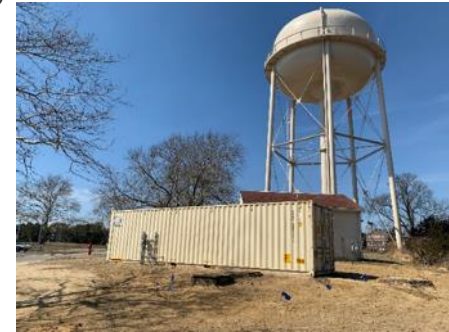
Mobile (40' CONEX) IX Treatment System. Connected to existing backup supply wells and water tower
