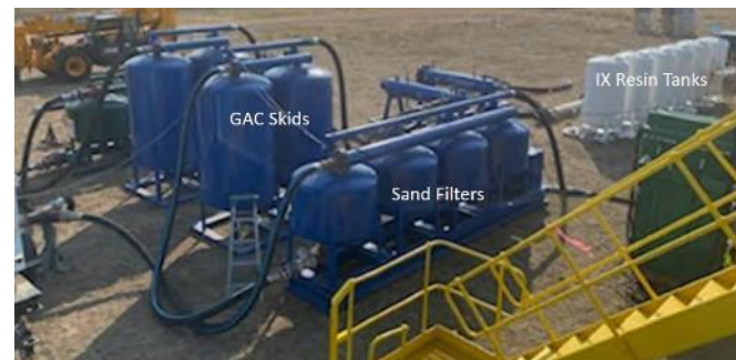
Water treatment system
