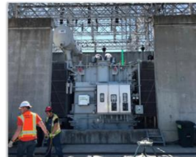
John Day Transformer Replacement
