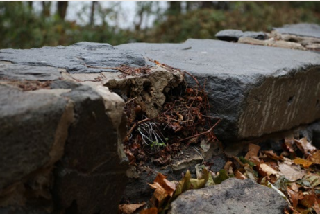
Current: Deteriorated stonewall
