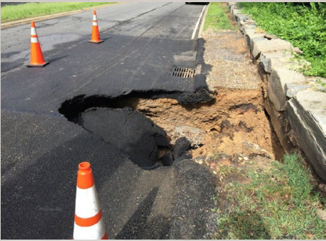
May 2019 major sinkhole
