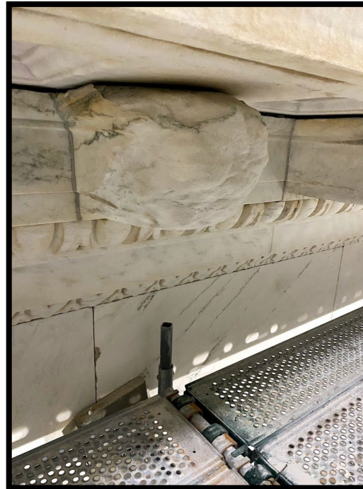
Modillion Existing Condition
