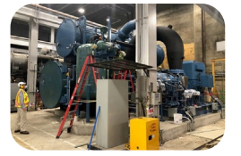
Refrigeration Plant Revitalization
