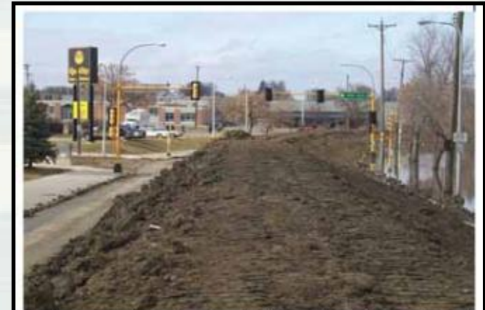
An Emergency Levee Protects the City at Second Street during the 2001 flood.
