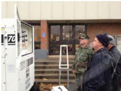
Hurricane Sandy 2012, CDR Marnell with contractors inspecting generators
