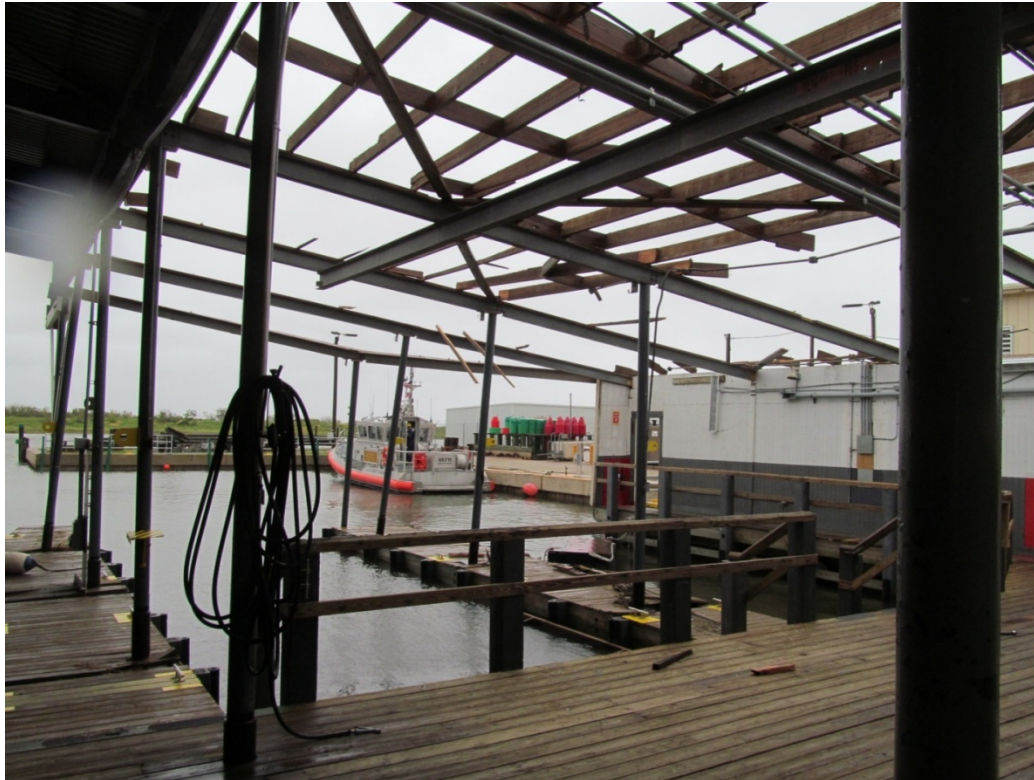
Port O'Connor – Roof Lifted off and loose columns
