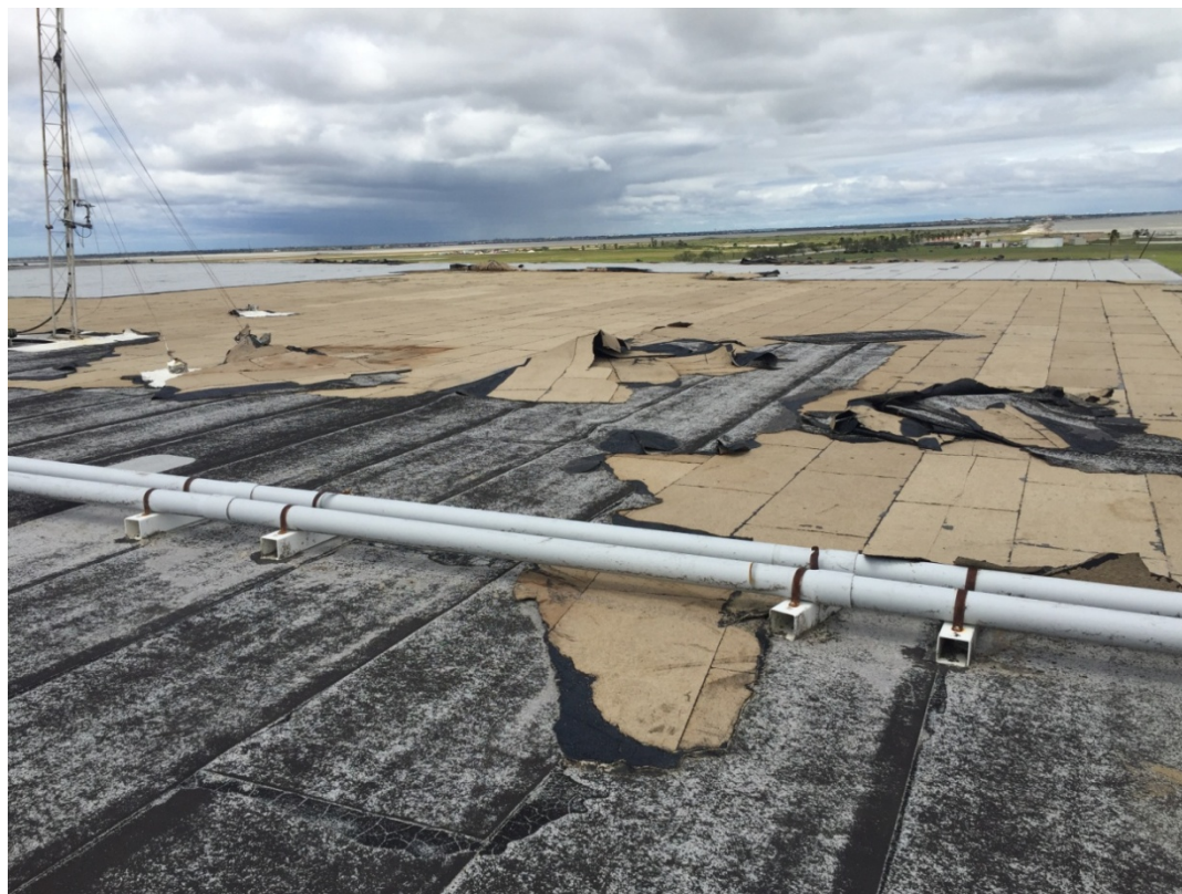
Corpus Christi - Roof membrane peeled back numerous locations.
