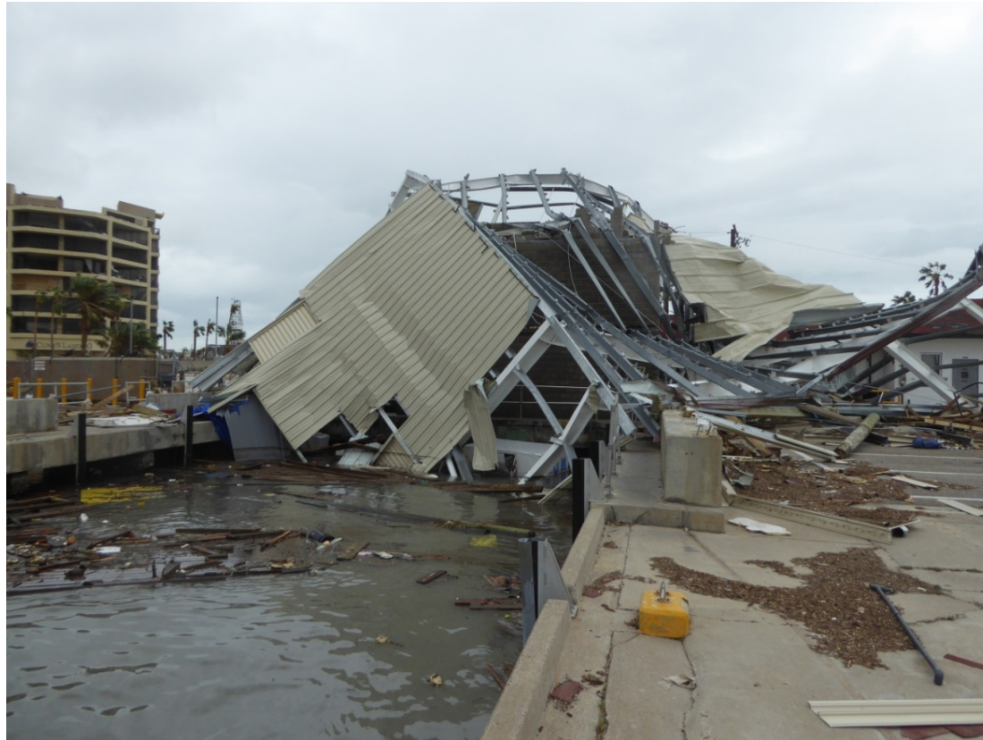
Port Aransas – Boat House Destroyed
