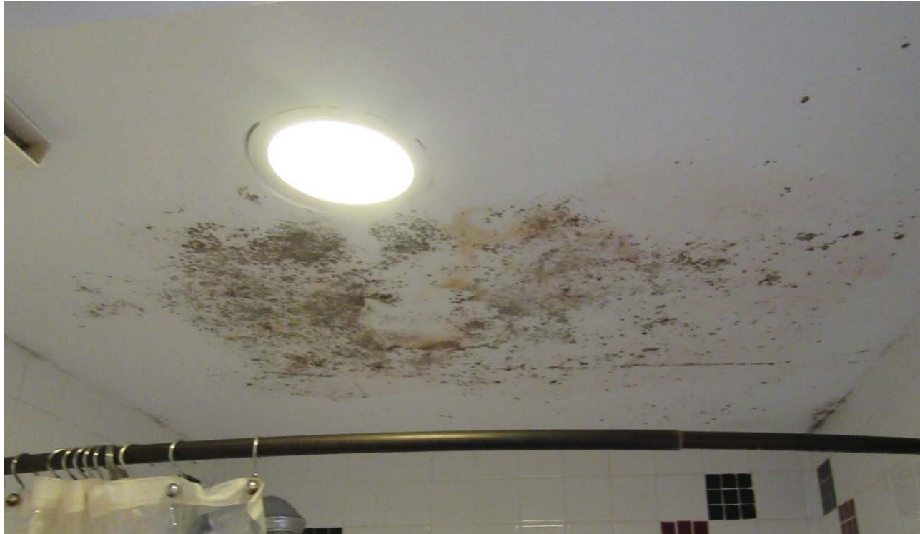
Bayamon Housing – Roof vent damage causing mold growth from water intrusion
