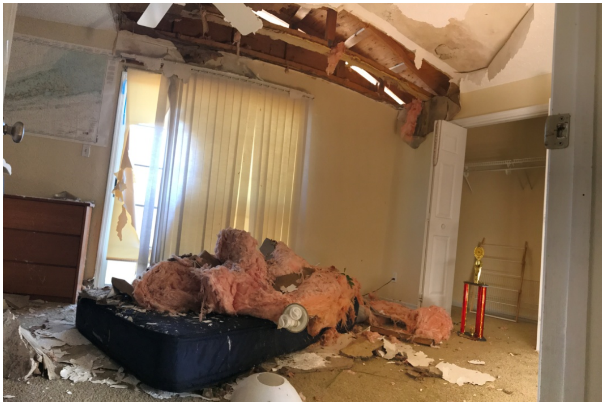
Marathon – Interior water damage to housing from the roof
