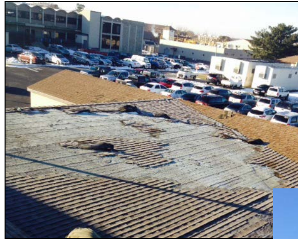
Roof Damage Cape May, NJ
