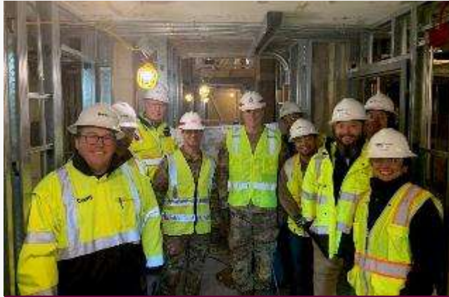
D/B Fort Bragg Barracks Renovation Owner: USACE Omaha (RDI) Location: Fort Bragg, North Carolina Value: $69,364,902
