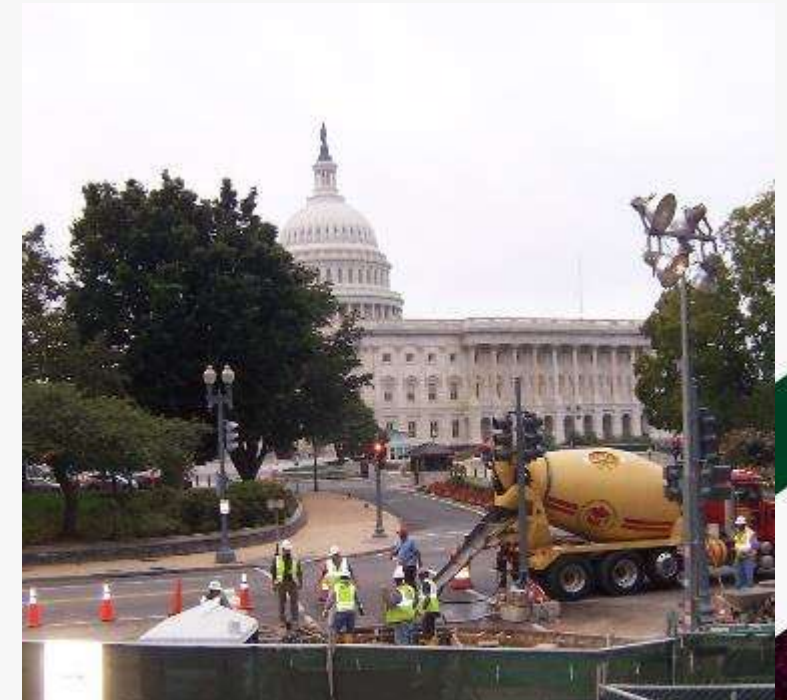
Senate Park Perimeter Security Owner: Architect of the Capitol Location: Washington, DC
