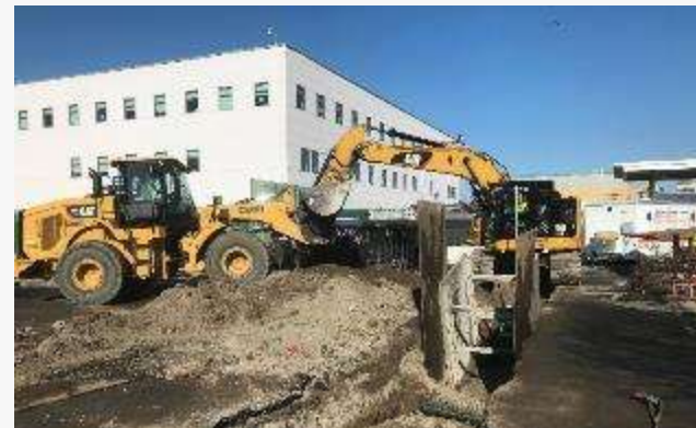
Jersey City Med Center Flood Control Owner: RWJ Barnabas Health (FEMA) Location: Jersey City, New Jersey Value: $35,056,313
