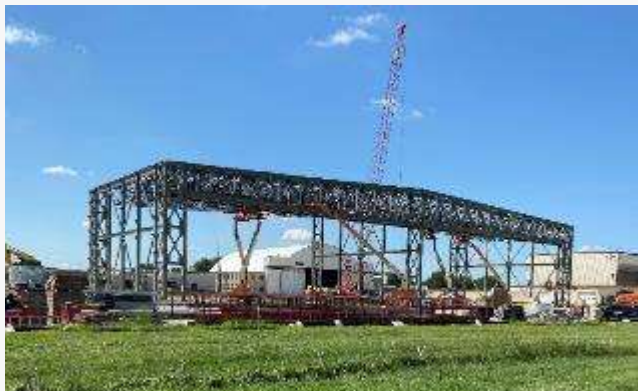
F-35 Fighter Alert Shelter Owner: USACE Omaha Location: Truax Field, Wisconsin Value: $20,243,914
