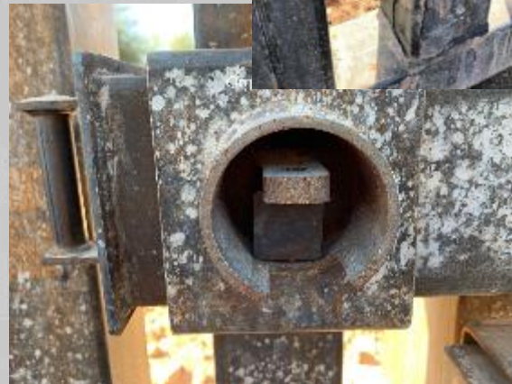
Locks removed from vandalism
