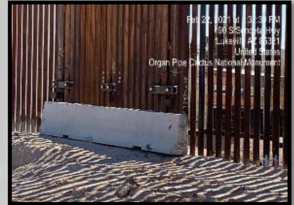
Jersey barrier placed in front of drainage gates by CBP (Tucson 2 - Lukeville Area)
