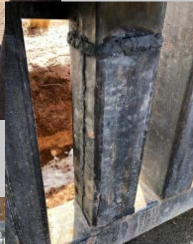
Bollard breach at Tucson 1
