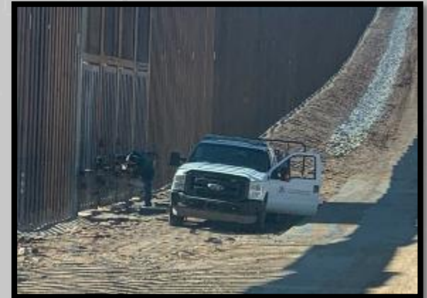
CPB welding drainage gates in the closed position (Tucson 3 - Douglas Area)
