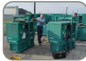
Emergency Power (249 th Prime Power Battalion)
