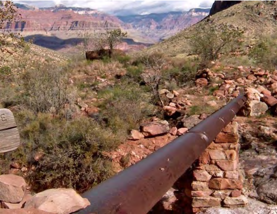
Trans-Canyon Water Distribution Pipeline, Grand Canyon National Park, AZ
