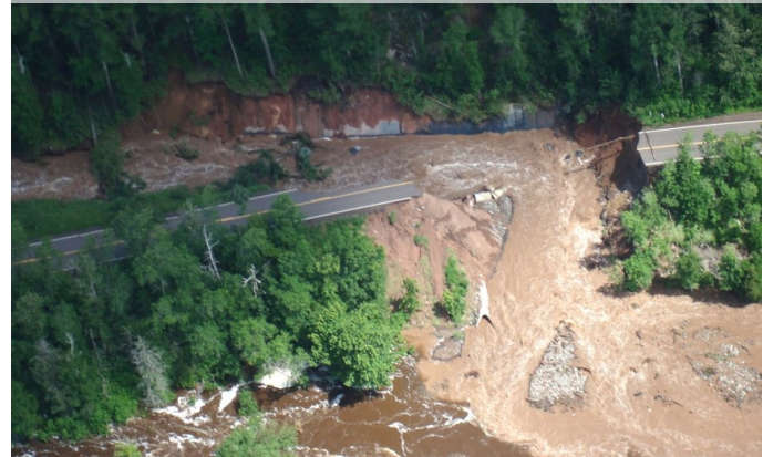
Hwy 210 Washout near Jay Cooke State Park (photo courtesy of MnDOT)
