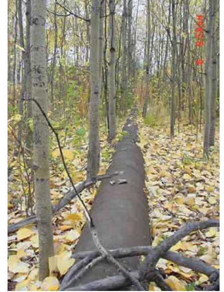
Haines to Fairbanks Pipeline. Photo DEC.Alaska.Gov.
