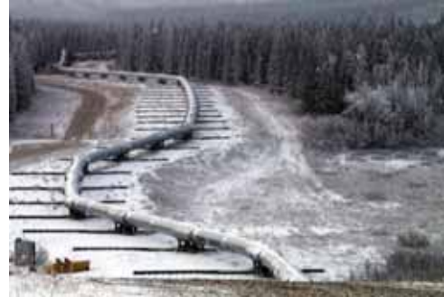
The pipeline includes slider supports where it crosses the Denali Fault.
