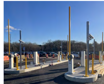
Authority-Wide Parking Revenue System Installation and Upgrades (Braintree LEX)
