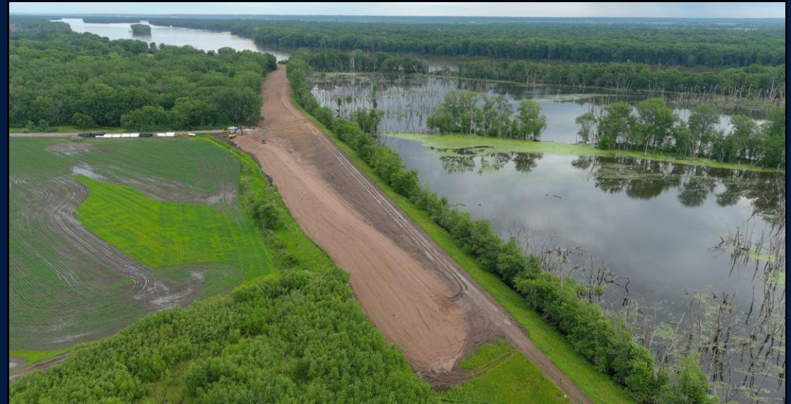
Rough Grading of the Muscatine Island Levee prior to HydroTurf Installation, June 2024.
