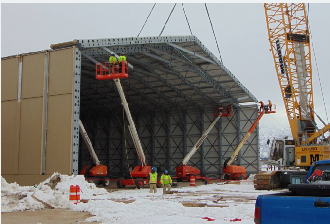
A prefabricated roof element being lifted onto the Hill Air Force Base's F-16 maintenance hangar. Courtesy of ADS Inc.
